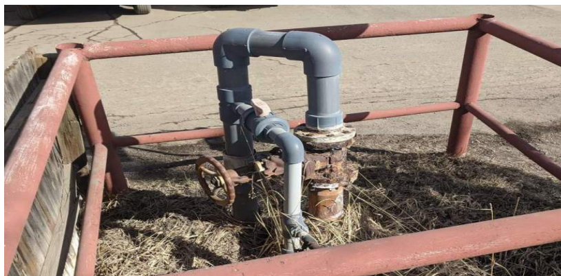
Figure 3. Corroded Well Head
