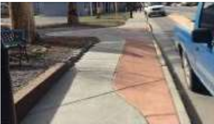
The colored concrete will be made steeper to widen the sidewalk. The driveway and wavy sidewalk to the west will be replaced with a standard CDOT driveway.
