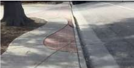
The curb height will be increased here to widen the sidewalk. The driveway to the west will be replaced with a CDOT standard driveway.
